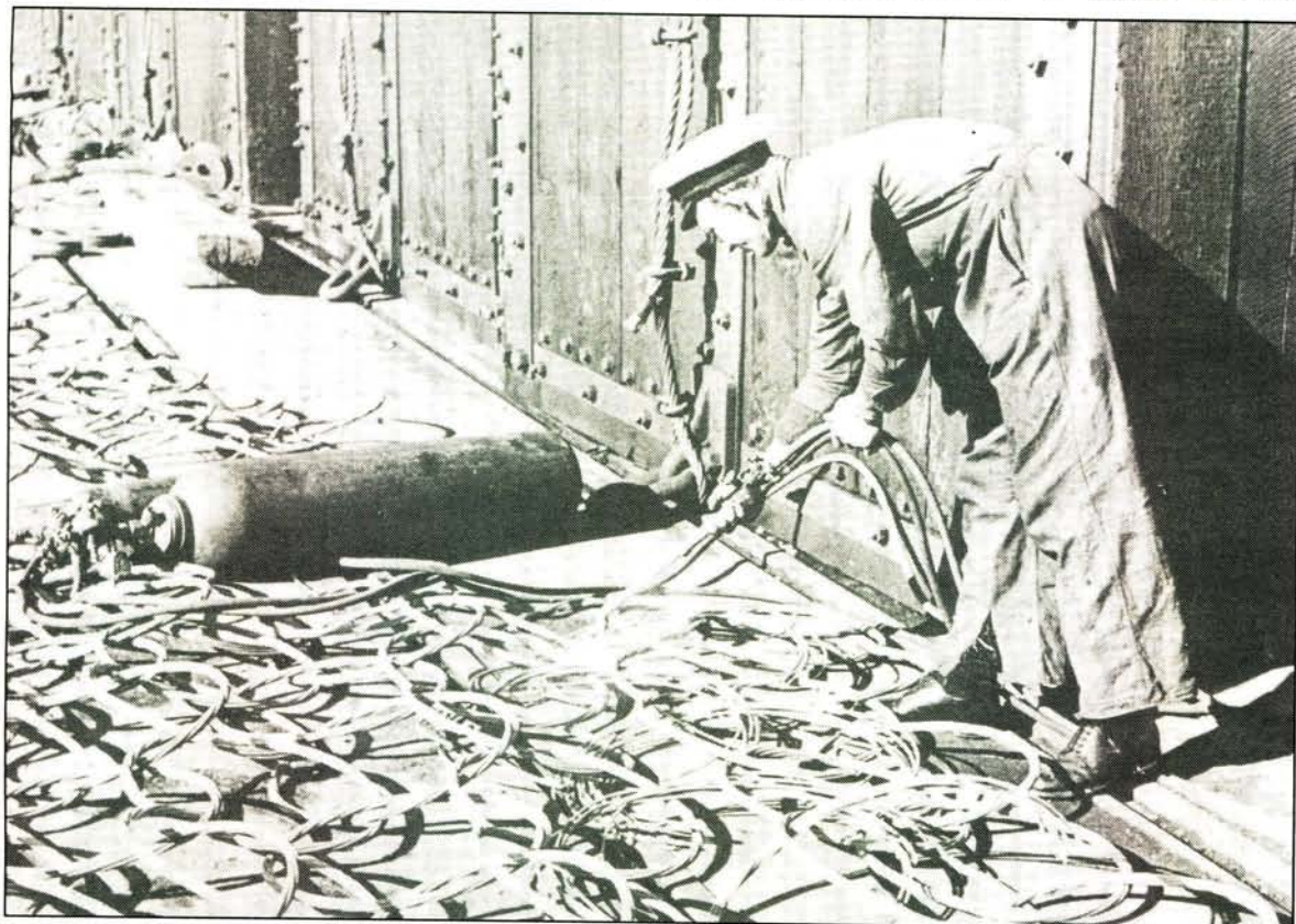
Oxy-acetylene cutting was the quickest method of removing broken or distorted grommets from an anti-torpedo net.
