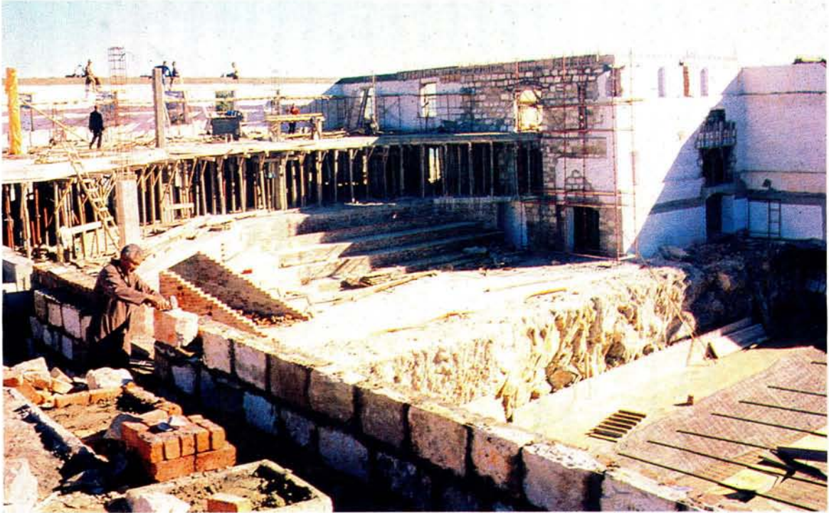
Restoration of the Old Mill at Mossel Bay to house the new maritime museum. In the foreground excavations are underway for space to house the replica caravel (Photograph: South African Panorama)
